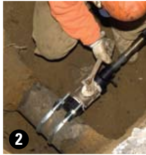
2 Open corp stop valve.
