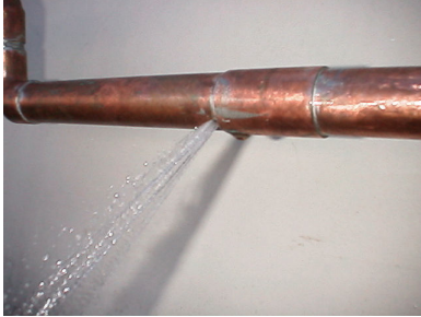
Leak at solder joint in copper pipe.
