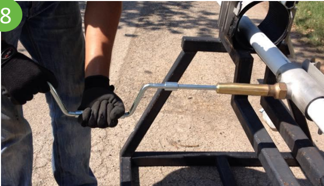
Tap through Corporation Stop using a VegaDrill for best results on plastic pipe.
